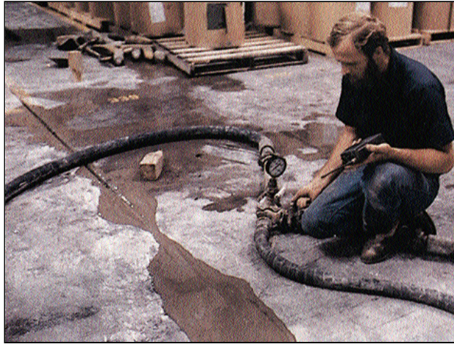
Figure 3. Undersealing grout appearing at joint edges shows that voids under the slab have been filled.
