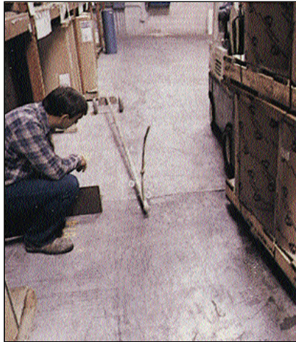
Figure 1. Deflection measurements are taken as a loaded forklift crosses over a joint. Too much deflection means floor life will be shortened and maintenance costs will be high.
