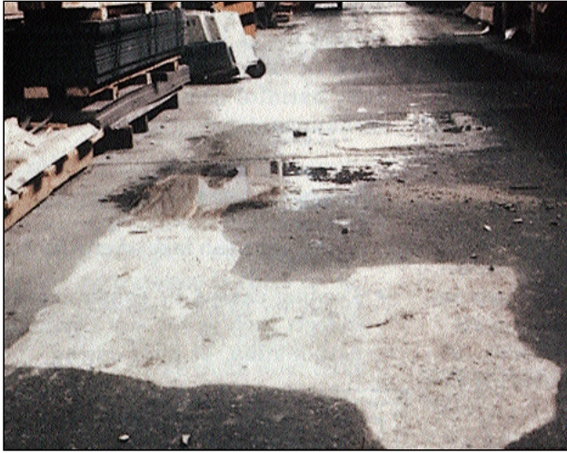
Figure 7. Coatings won't fill in eroded or badly spalled areas. A topping or overlay is needed.
